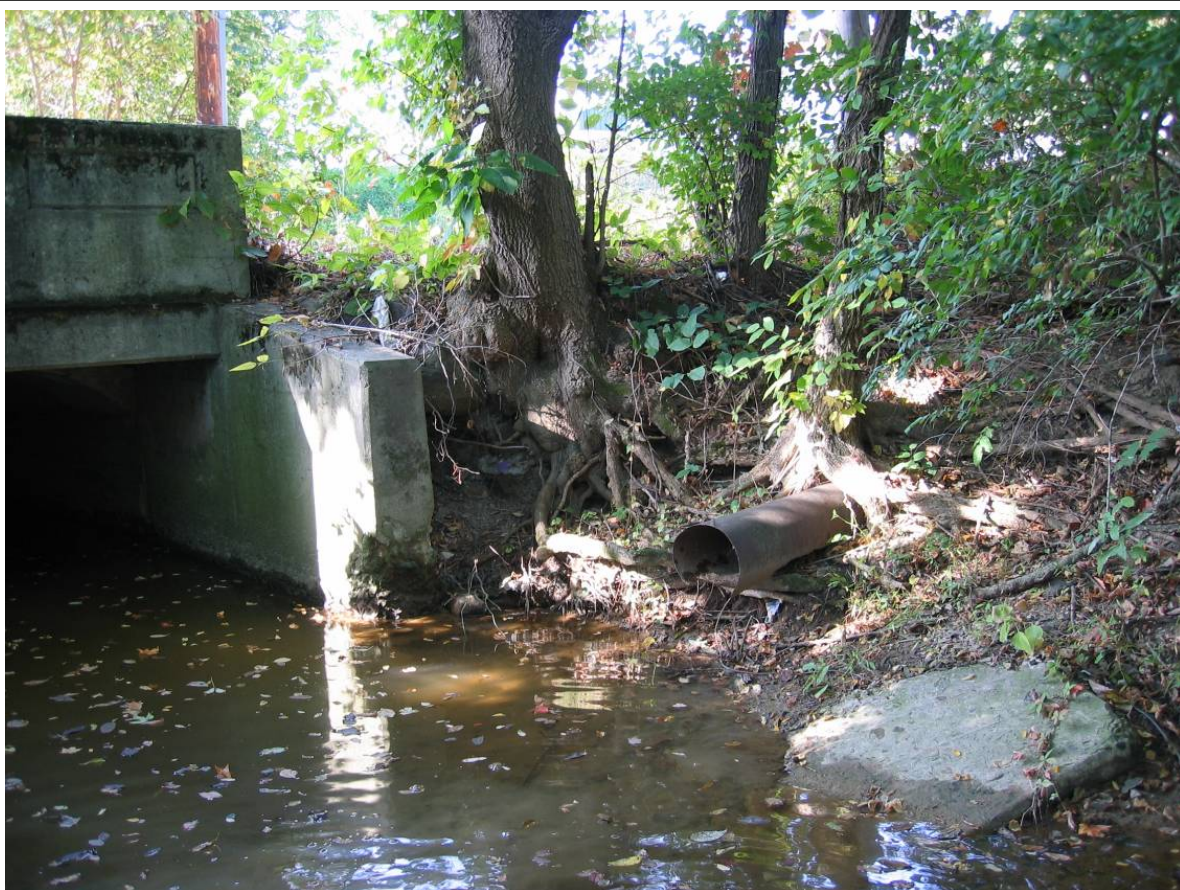
Figure 3. Numerous pipes empty into Warm Springs Run, a highly impaired stream.
