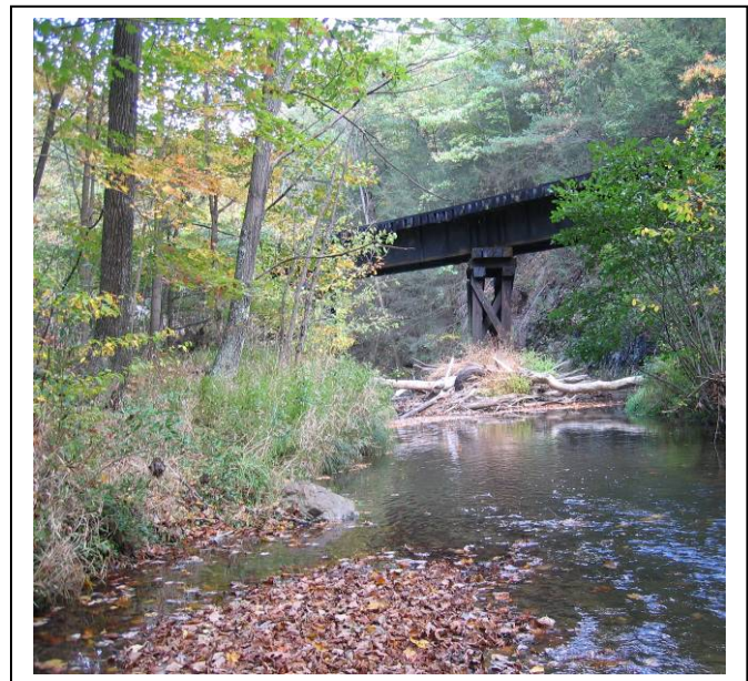
Figure 11. Debris jam and channel alteration caused by the railroad bridge in Section 7.
