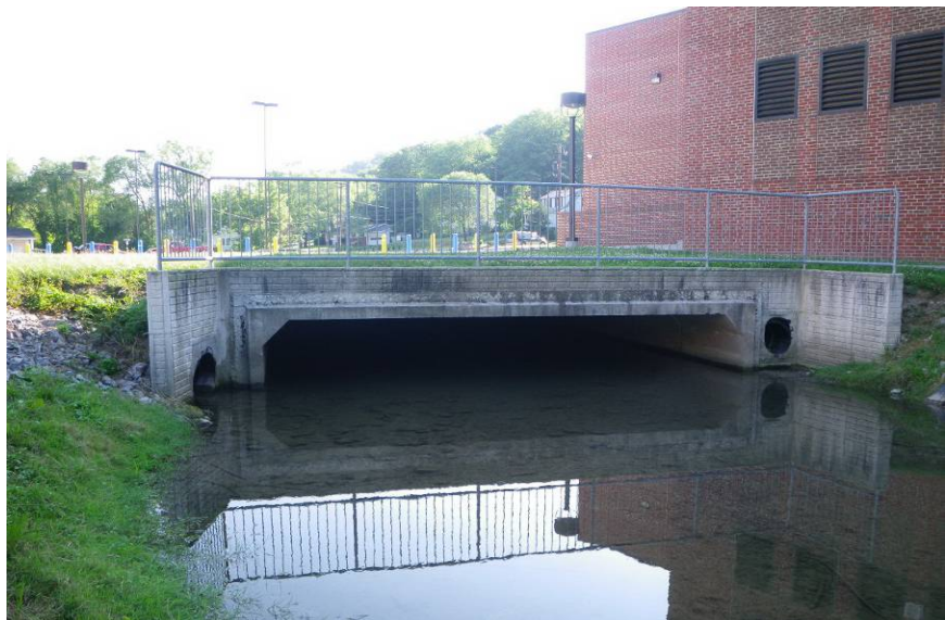
Figure 32: Closed culvert increases the sediment load, exacerbating flooding
