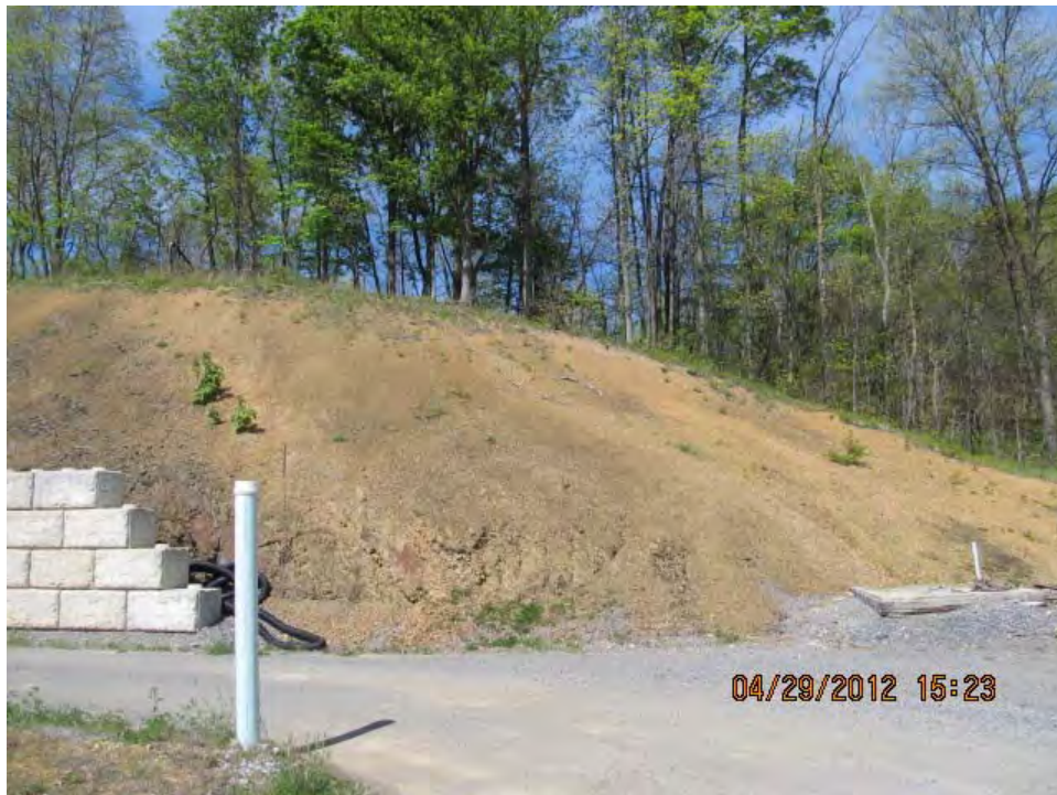
Figure 28. Exposed weathered shale behind shopping center. Slope devoid of vegetation.
